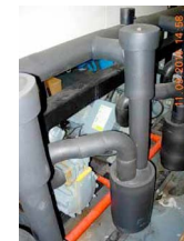
Above: Pipe Insulation
