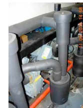
Above: Pipe Insulation
