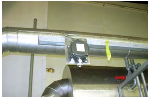
Refrigerant leak detector in a compressor plant room
