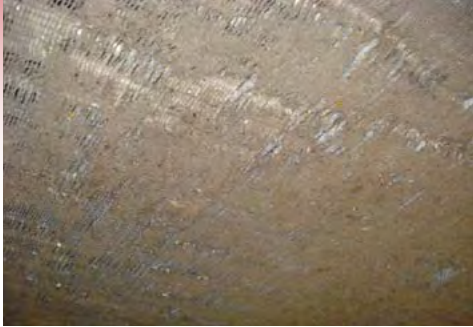
Build-up of debris on a condenser.
